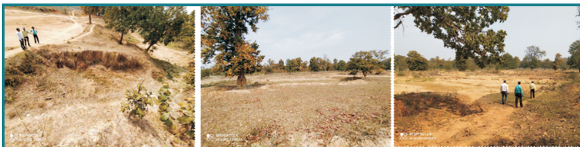
Fig. 3 In Pavan mine photographs of sagging area(left) a large area subsided, trees are also tilted due to deformation(middle and right) due to mining and dislocation of surface strata of Rajgamar coalfield of Chhattisgarh.
